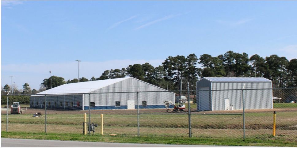
Figure 9: Exterior view of the new STEM building under construction, March 11, 2026. Photo by OSA.
